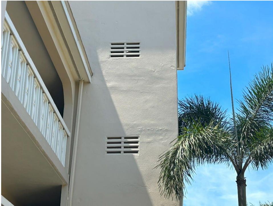
19. Example of stucco EFIs with no control joints which is resulting in cracking.
