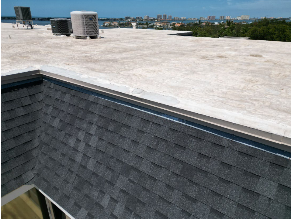
7. View of the membrane peeling along the top flat roof on the south side.
