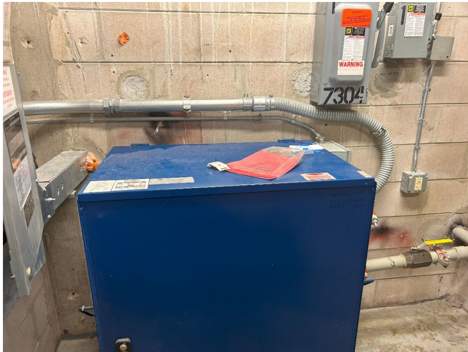
32. View of a portion of the elevator equipment.
