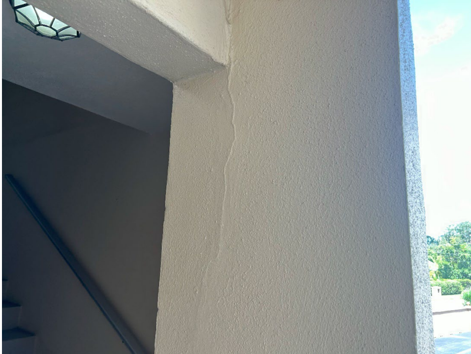
29. The shear crack propagating from the beam in front of Unit 110 should be exposed in a Phase 2 investigation.
