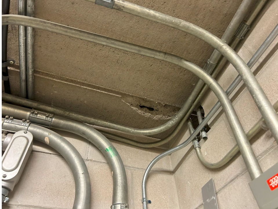
25. Spalled concrete in the electrical room is exposing rebar to the elements. This rebar should be exposed to confirm how much corrosion is present in a Phase 2 investigation.
