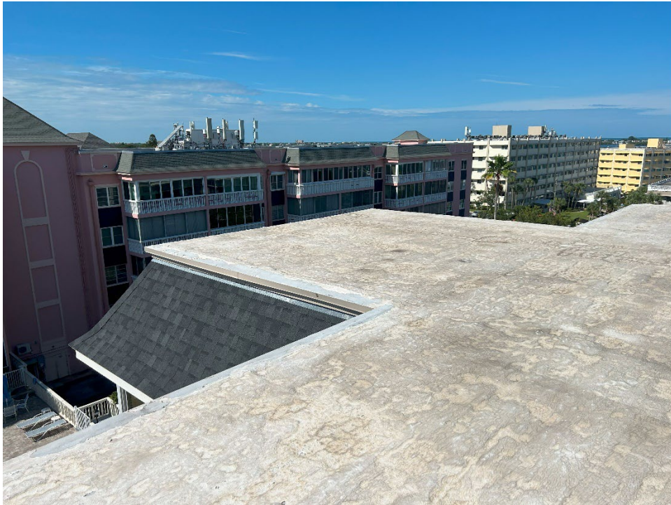
4. View of the membrane peeling along the top flat roof.
