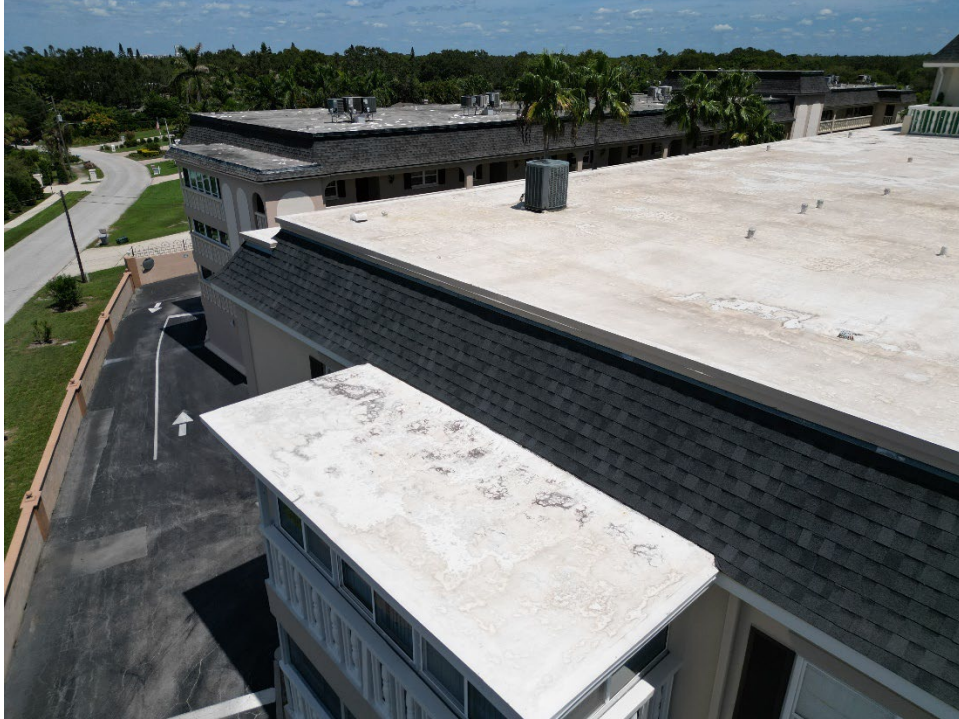
11. An example of significant deterioration on the TPO roof is the west flat roof.
