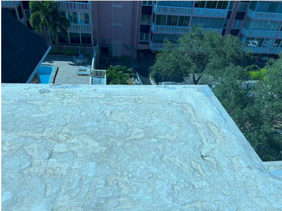
6. View of the membrane peeling along the top flat roof.
