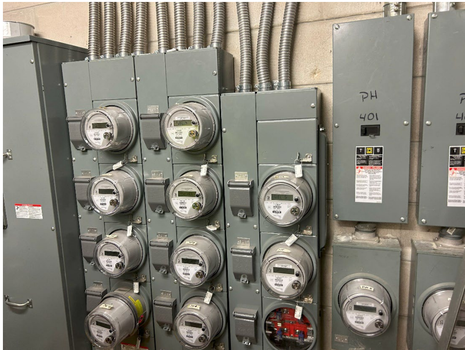
33. Example of the main electrical system conduits and meters.
