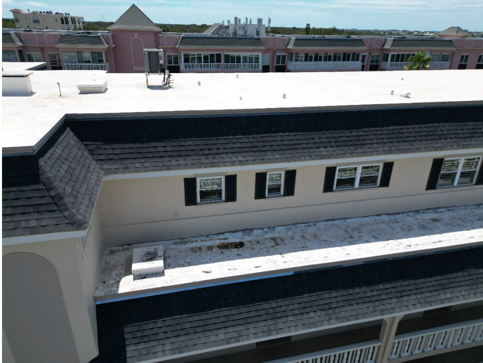
9. An example of significant deterioration on the flat roof, along the north side of the building, on the lower west flat roof.
