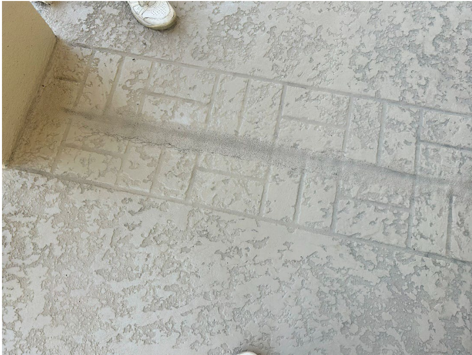
16. Cracks are occurring at the control joints in the breezeways, due to the age and design of the joints.
