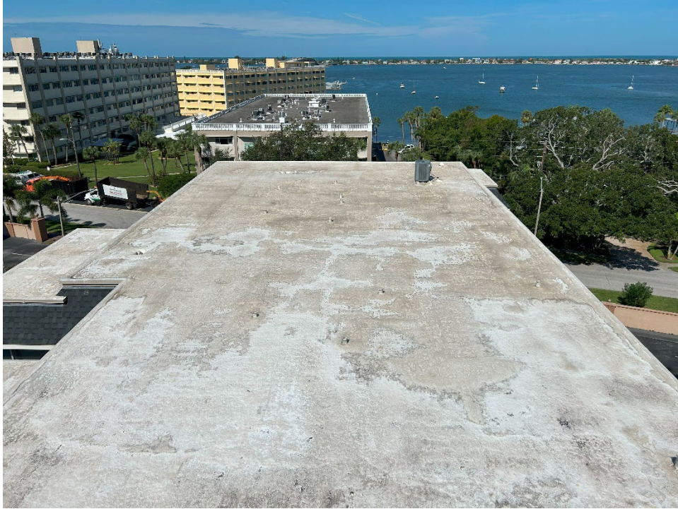
5. View of the membrane peeling along the west lower flat roof.
