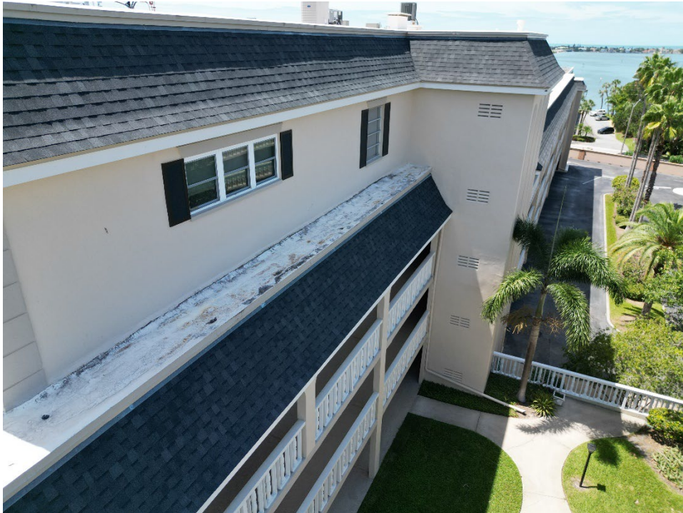
8. An example of significant deterioration on the flat roof, along the north side of the building, on the lower east flat roof.
